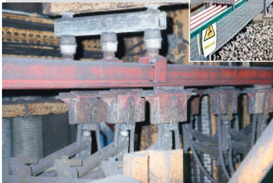
300 metres of 800A bar ↑ → with medium heat cover feeding two steelwork cranes. Dusty, corrosive and hot (+80°C) environment. Using insulated hanger clamps supplied pre-fitted to support brackets.
